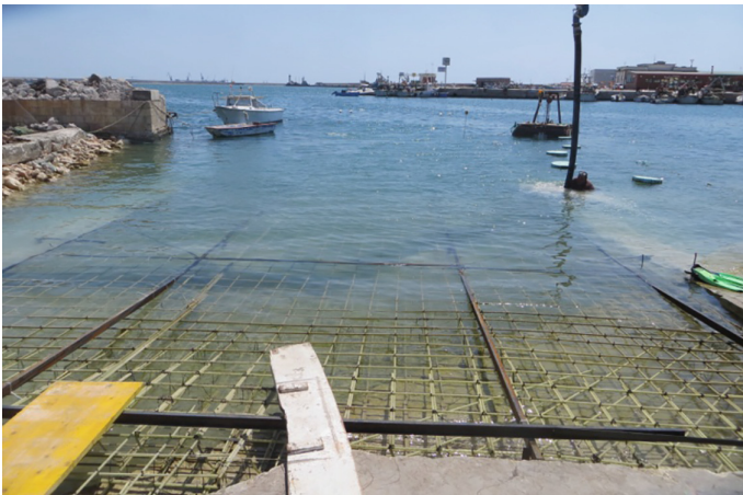
Fig. 12. GFRP cage installed under sea water. Diver casting concrete on the right side
