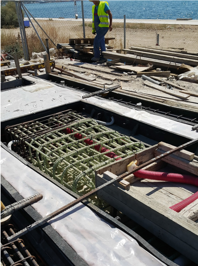
Fig. 1. GFRP reinforcements installed in a section of the Athens tram track beds
