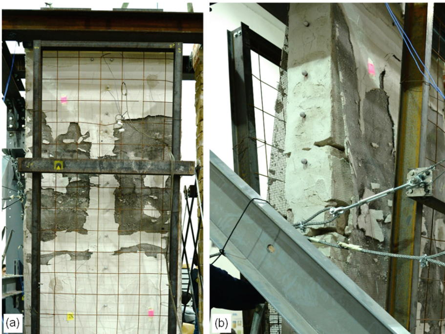
Fig. 3. Damage pattern on the stone wall retrofitted with BFRM at the end of the shake table tests.
