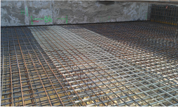
Fig. 14. Section of slab reinforced with GFRP cage that splits the steel cage
